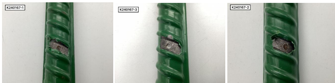
Details disbonded area
