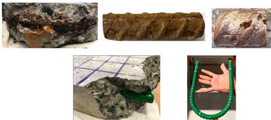
Plate 3. Visual inspection of corrosion conditions of BB, ECR and ECRCD in concrete blocks and after retrieval
