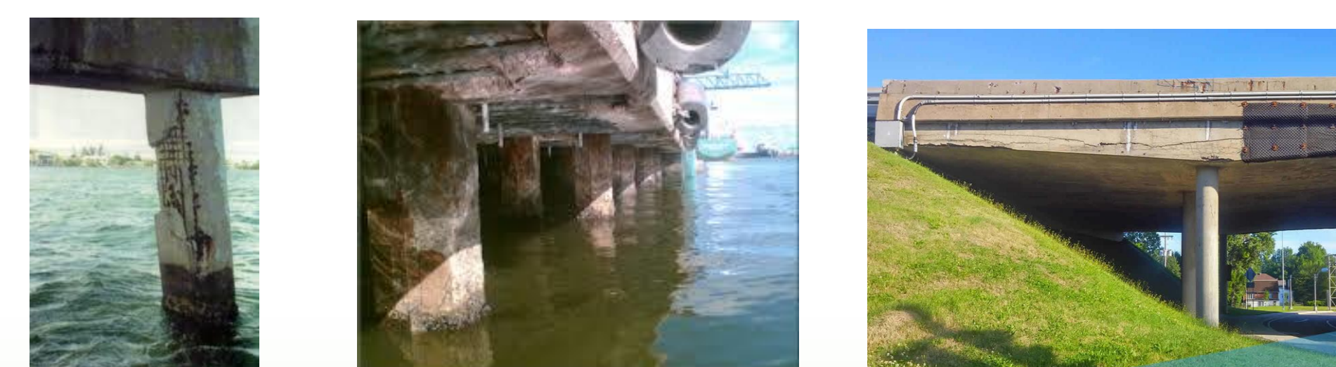
Figure-1 Damage caused by steel corrosion to reinforced concrete structure
